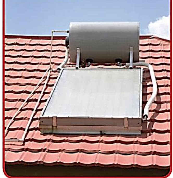
A photovoltaic (solar) panel
